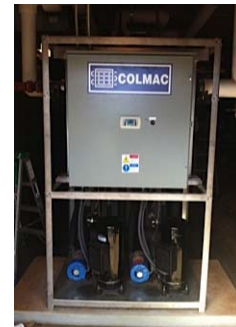
Colmac Model HPW24 installed at Kukui'Ula on Kauai. Mahalo to Beall & Assoc. and Commercial Plumbing
