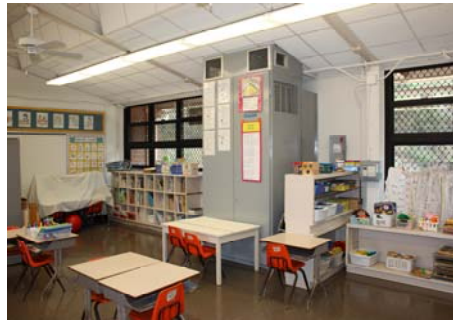
Marvair Scholar A/C. Inside Classroom at Lincoln Elementary School on Oahu
