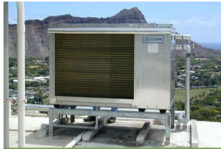
Colmac Air Source Heat Pump in Waikiki
